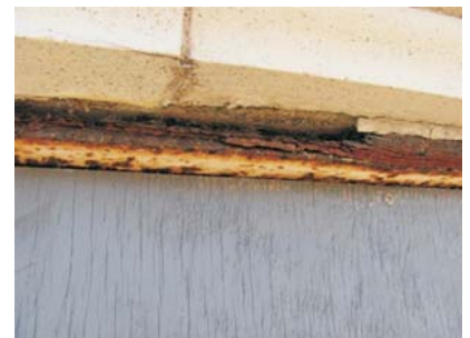
Image 8. Severely corroded lintel
