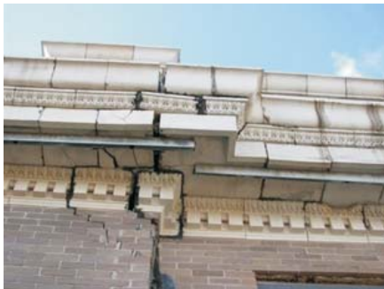
Image 7. Temporary reinforcing previously added at displaced terra cotta
